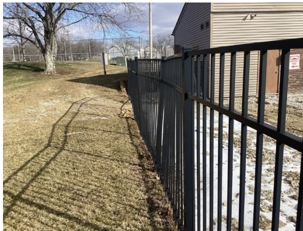
Fence leaning section
