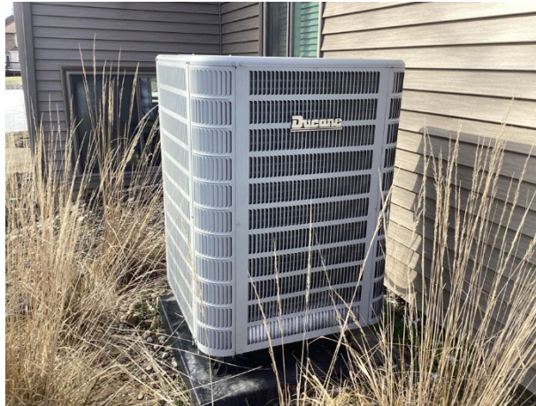
Split system condensing unit
