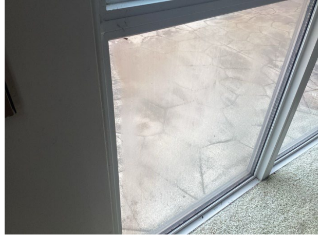
Evidence of broken seal
