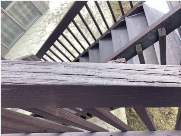
Railing wood split
