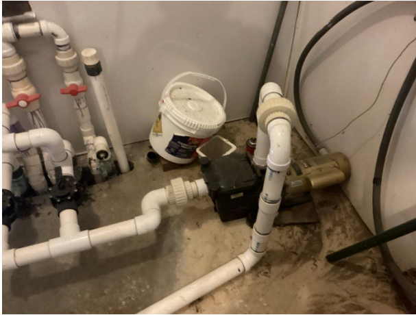
Pool mechanical equipment
