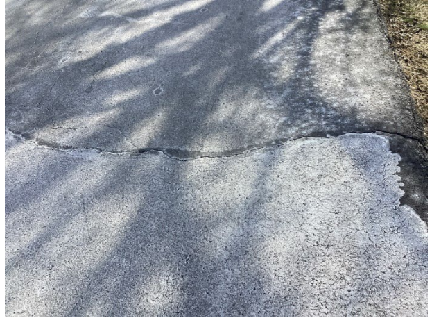
Street pavement crack
