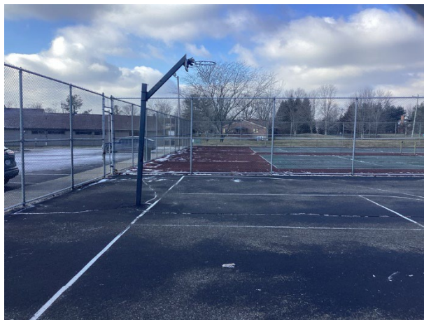
Basketball goal damage
