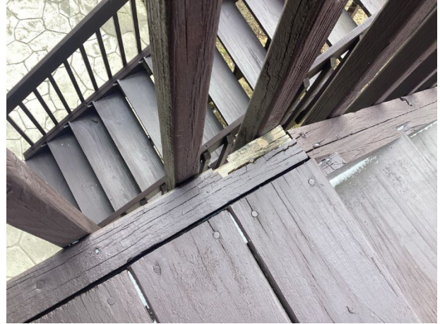
Deck board damage
