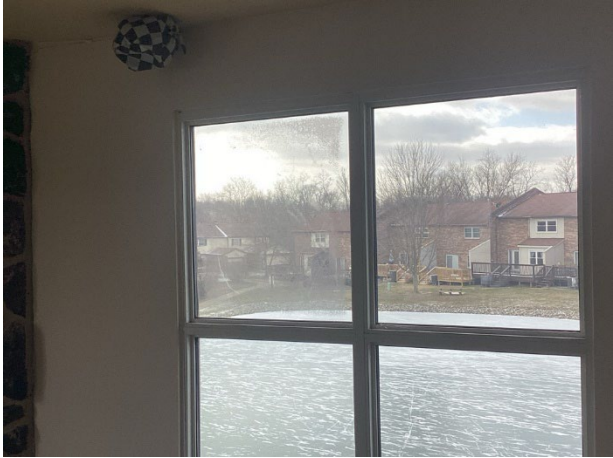
Evidence of broken seal
