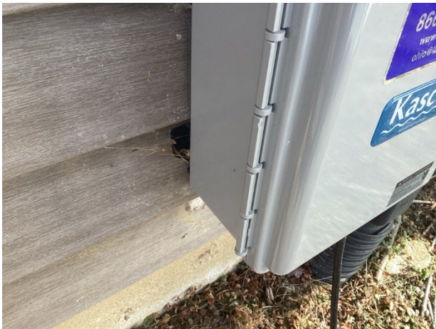
Gap in siding
