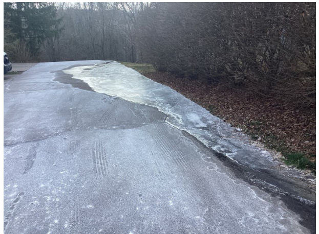
Standing water likely due to downspout discharge
