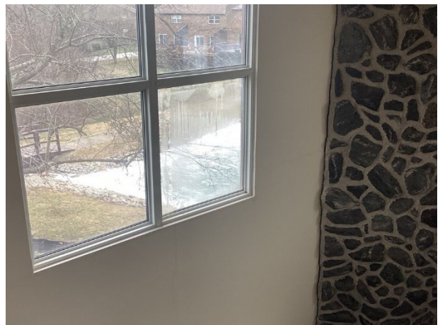
Evidence of broken seal
