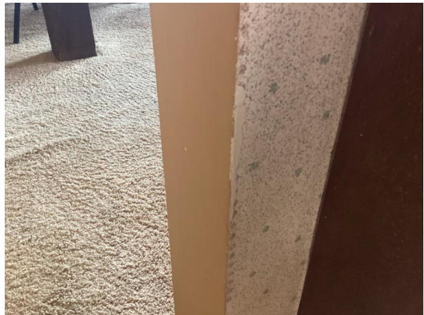
Wall covering damage
