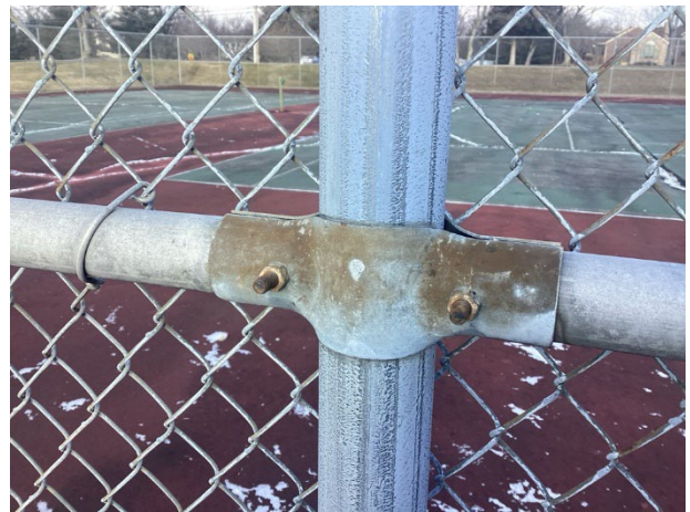
Fence finish deterioration
