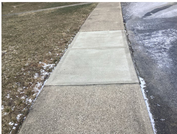
Sidewalk previous repair
