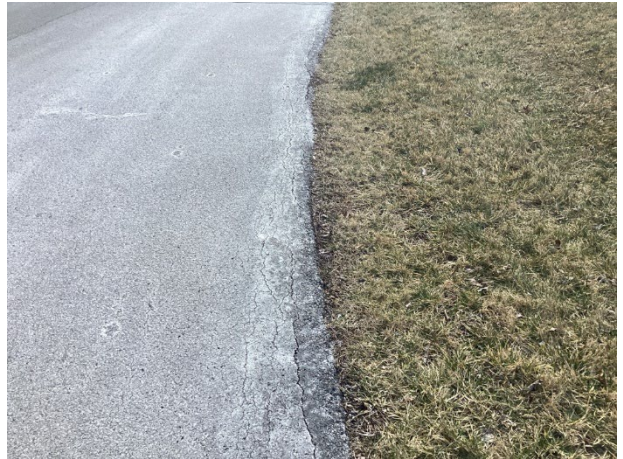
Street edge deterioration
