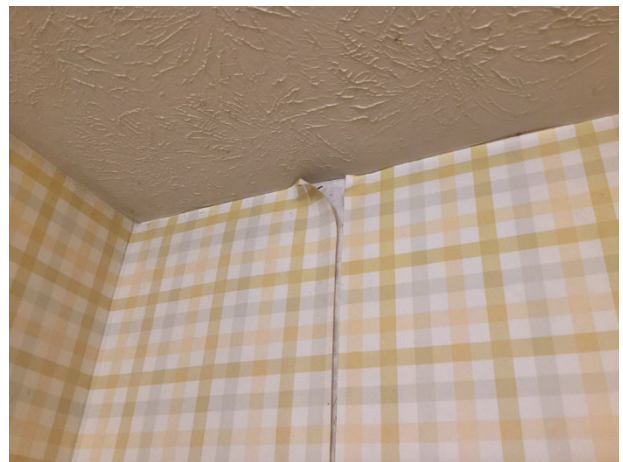
Wall covering seam adhesion failure
