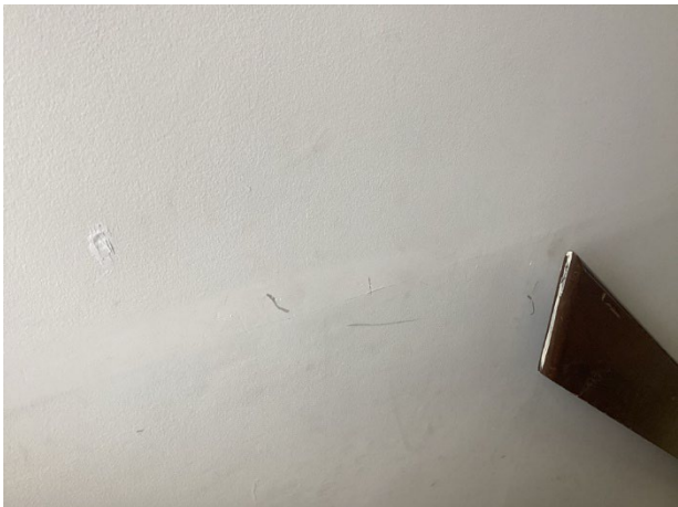
Wall scuffs and repairs
