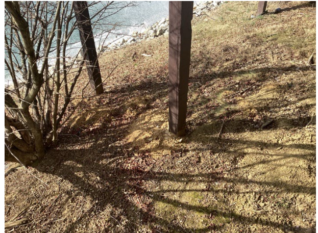
Wood post in contact with ground
